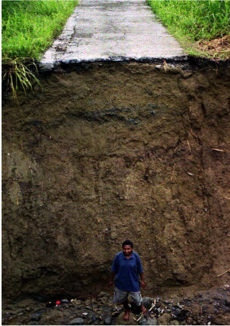
Plate 2.1. Collapsed culvert at Igora VOP, Popondetta
